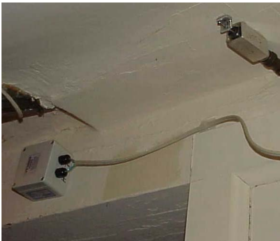
Figure 5.9 Weather and Stair Sensor
